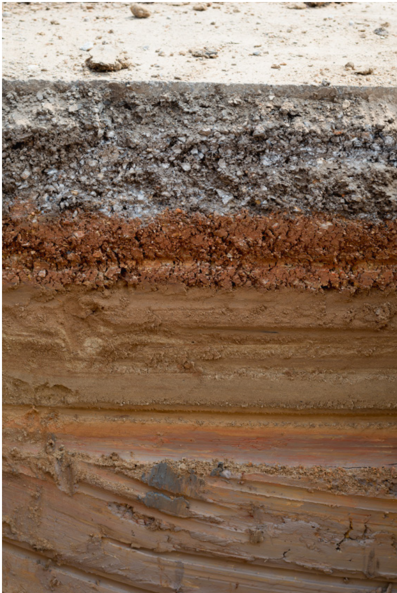
Asphalt and soil layers, with visible damage from water erosion. Credit: RachenStocker
